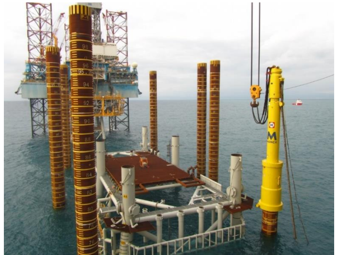
Figure 60. Typical offshore pile driving arrangements. Photograph courtesy of Mr P van Esch, Heerema.
