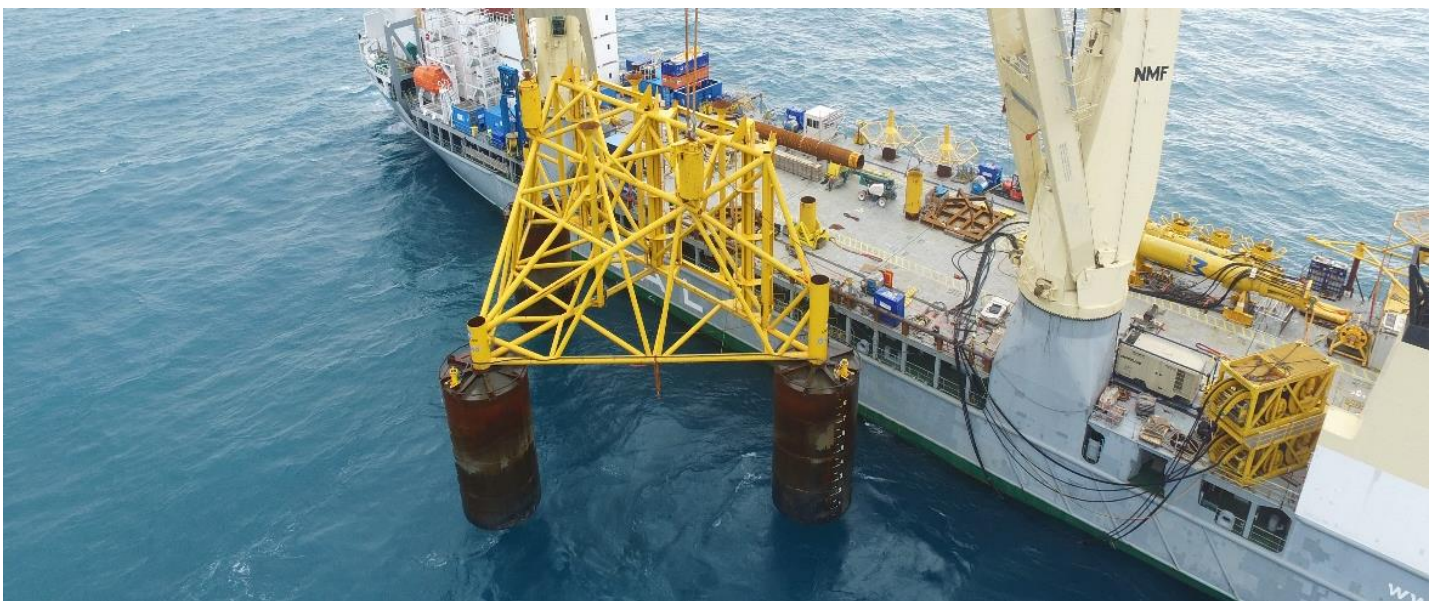
Figure 68. Deployment of suction-bucket supported pile guide frame required for driving of 1.5m diameter offshore piles in potentially loose Taiwan Strait sands, silts and low YSR very low I_p clays. Photograph courtesy of Ørsted.
