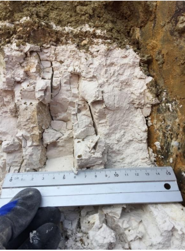
Figure 51. Putty and fracture zones of driving damage around Pile R2 after completing axial testing, also showing annulus of corroded steel at putty-to-pile shaft contact.
