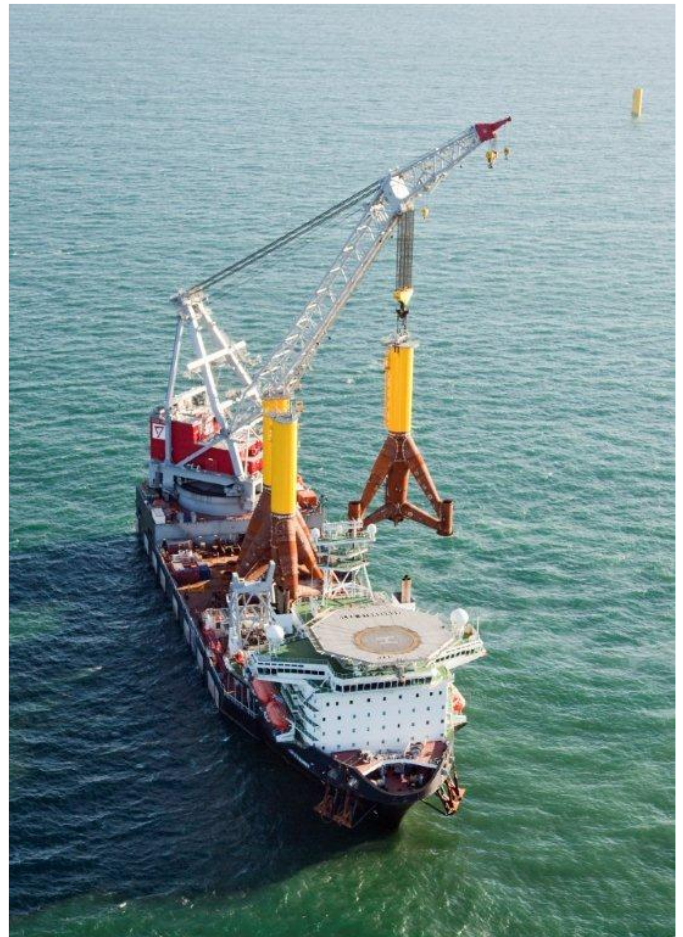
Figure 22. Installation of Borkum West 2 wind turbine tripods in 2011. German North Sea, photo by permission of Trianel.
